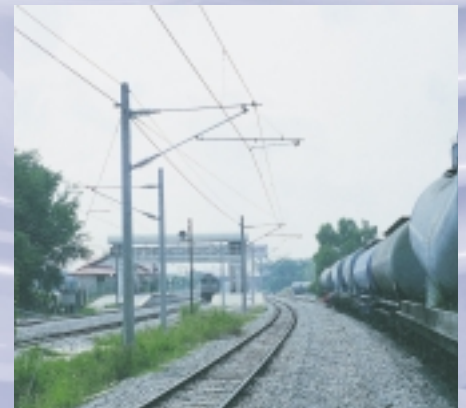
Tension and strut insulators in railway lines
