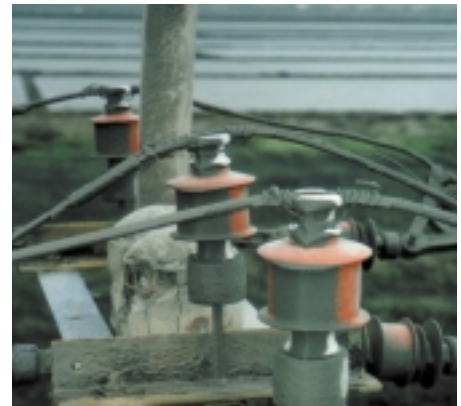
Working conditions of Raybowl insulators
