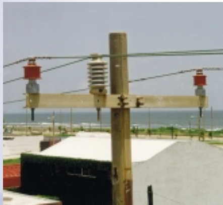
Raybowl insulators installed in a high polluted area in Latin America.
